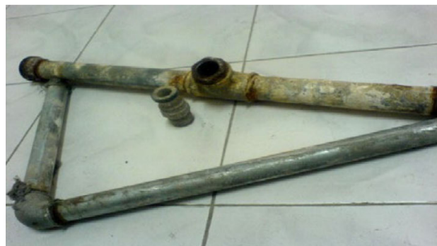
Fig. 1. Corroded aluminum pipes
